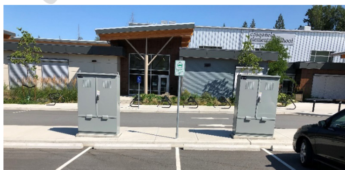
EV Chargers at ċasqanelā Elementary
